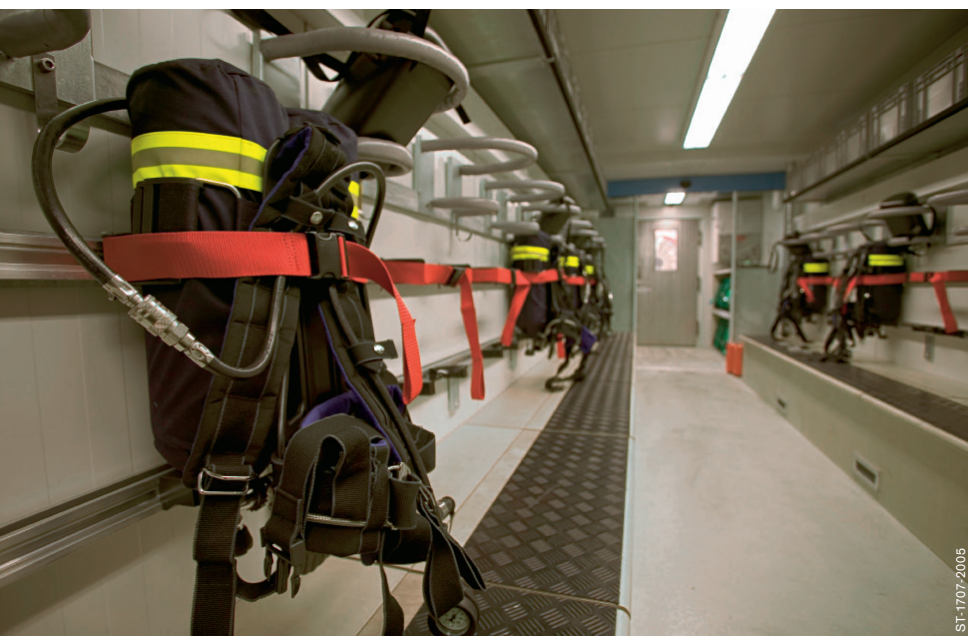
The rescue chamber is gastight so that occupants can breathe freely.
