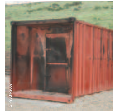
The Phase 3 system – three year old unit in use at the Los Angeles Fire Academy.
